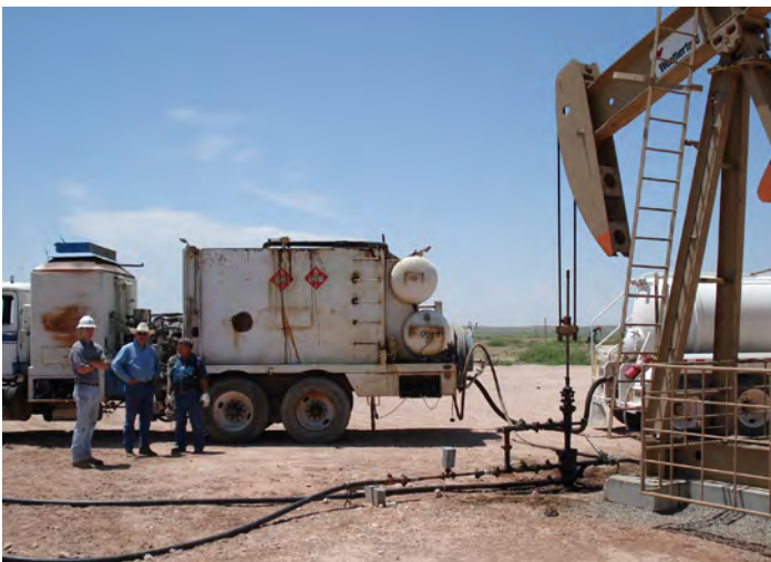
Pumper truck with diluted enzyme fluid followed by water truck to displace enzyme fluid into formation. (Chavez Co., NM)
